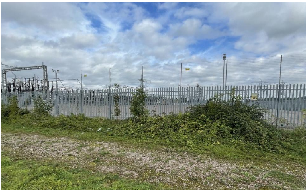
Image 3.10 Existing substation - Norwich Main 400 kV (Source: National Grid)
